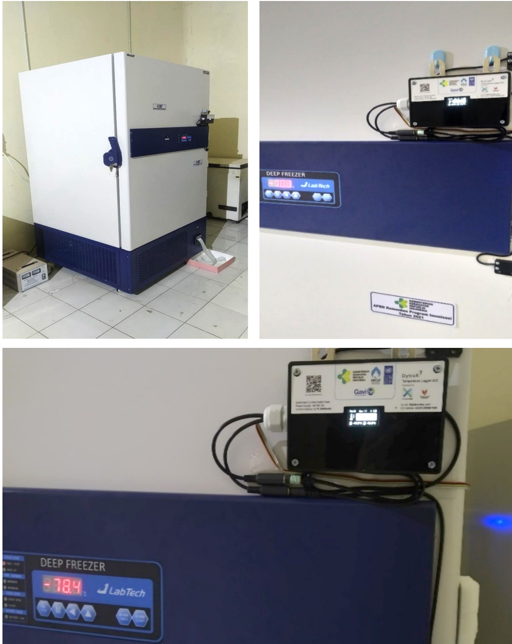
Figure 17. Temperature logger installation for Pfizer vaccine with a temperature of -90^{\circ} in Lampung City
